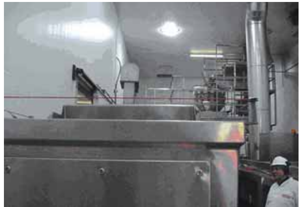
Note red pull cord, which does not prevent access
